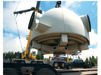
The nacelle of a decommissioned turbine is lowered to the ground. Fitzpatrick Mountain Wind, Nova Scotia.
